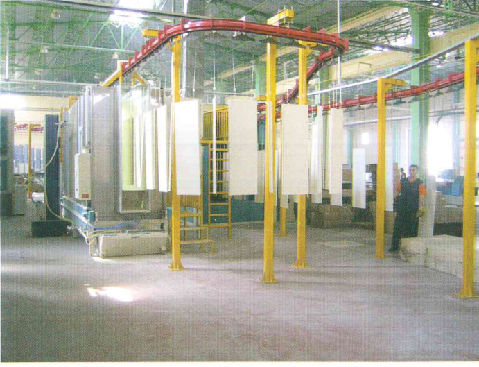
Market Reyonu Toz Boya Tesisleri Market Department Powder Coating Lines
