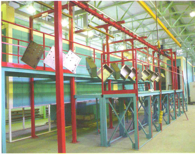
Elektrik Panosu Boyama Tesisleri Power Panel Painting Lines
