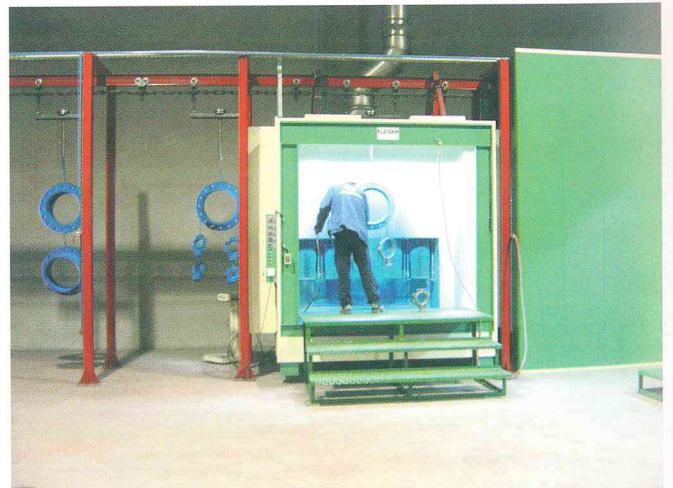
Vana Boyama Tesisleri Valve Painting Lines
