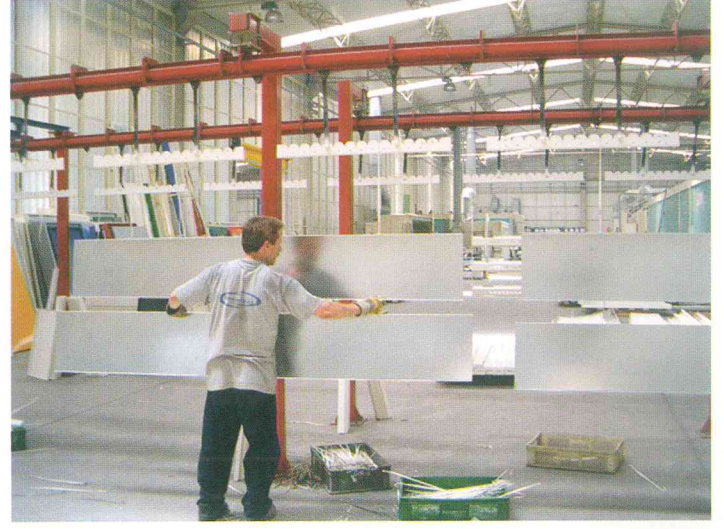
Market Reyonu Toz Boya Tesisleri Market Department Powder Coating Lines
